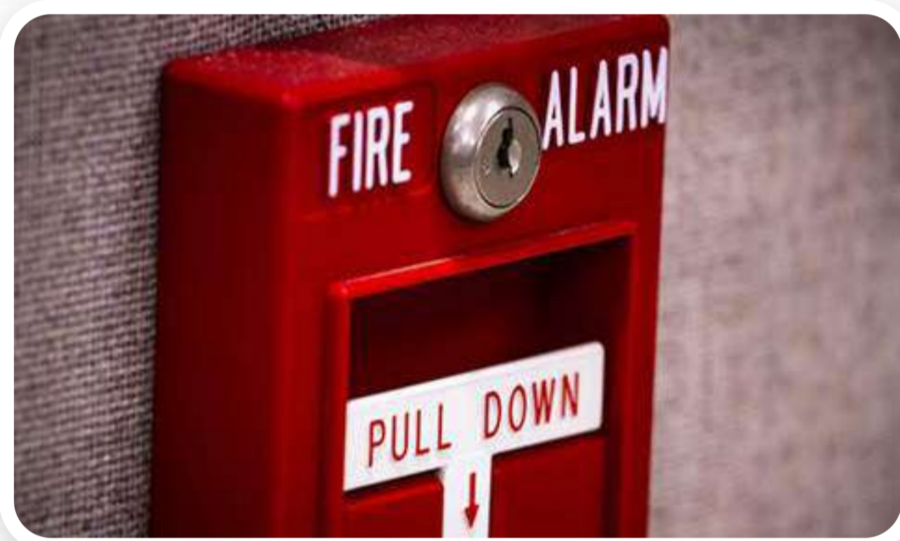
Fire Alarm and Detection
