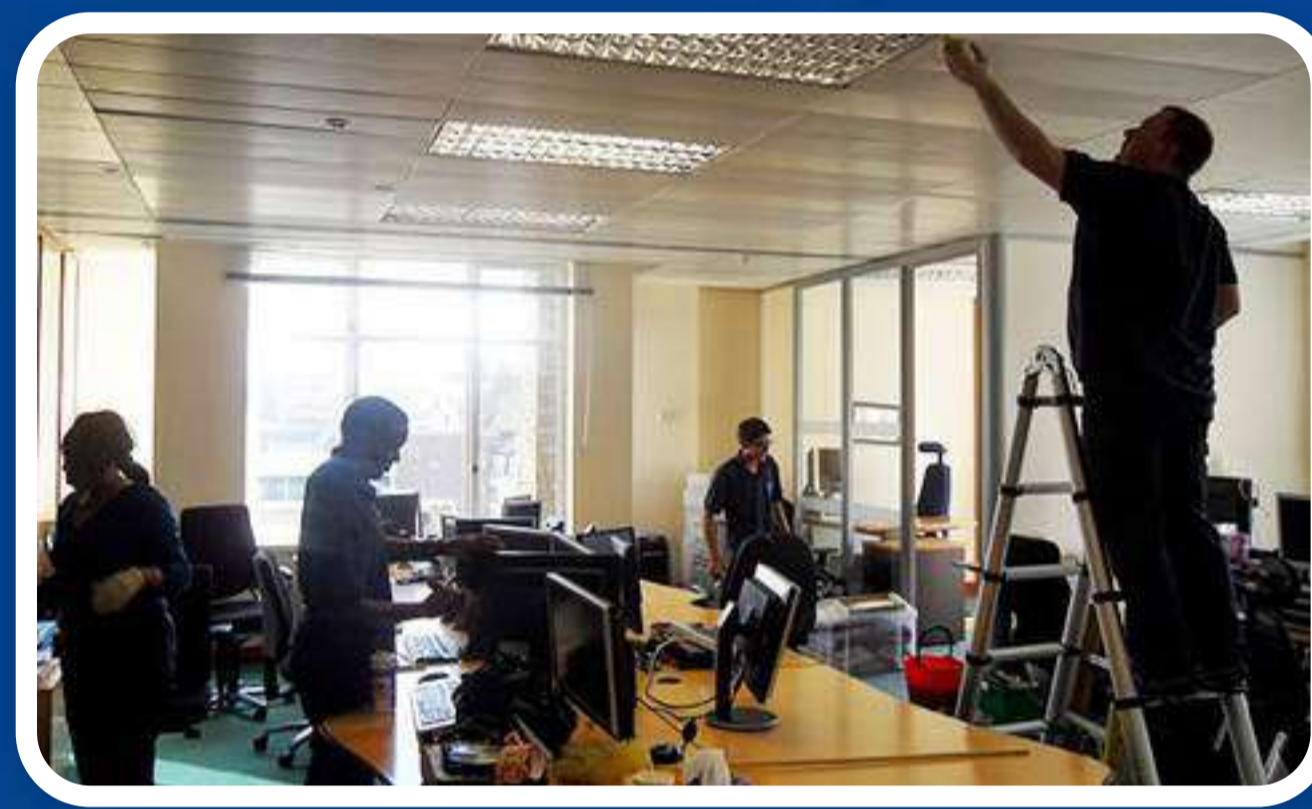
Building Management System AMC
